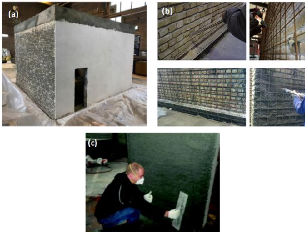
Fig. 2. (a) masonry building retrofitted with shotcrete [10] (b) brick walls strengthened with shotcrete [11] (c) strengthening of clay brick URM walls using Engineered Cementitious Composite (ECC) shotcrete [12]
